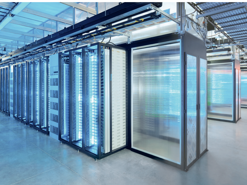
Evaporative cooling in the Meta (Facebook) data center in Luleå, Sweden
