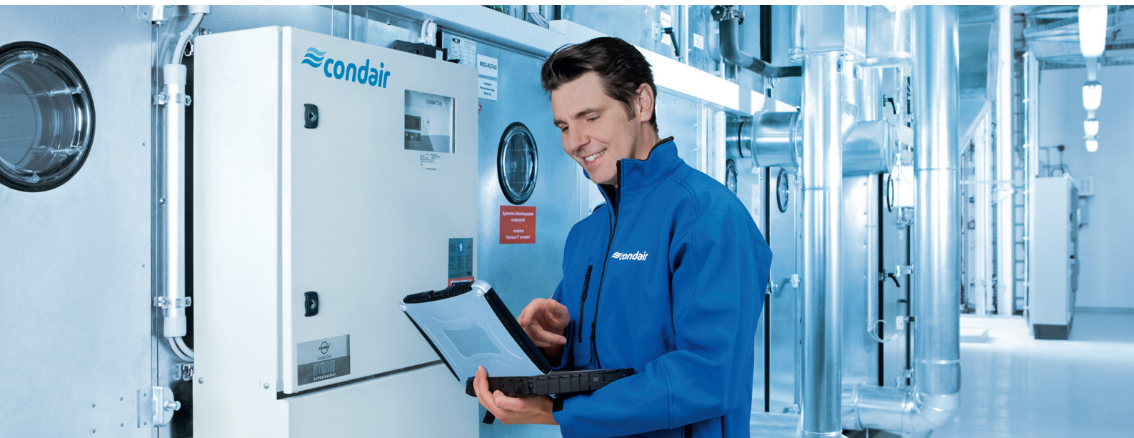
Condair DL in a ventilation and air-conditioning system
