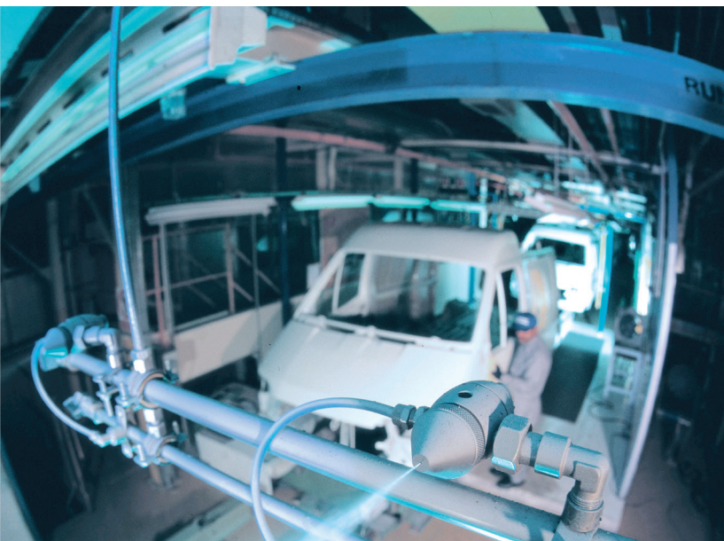
Humidification in an automotive paint shop
