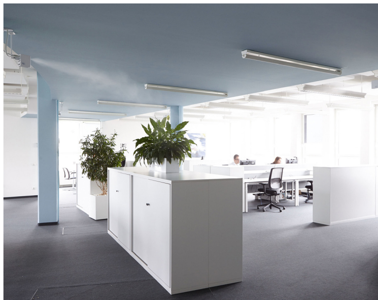
Humidification in an office
